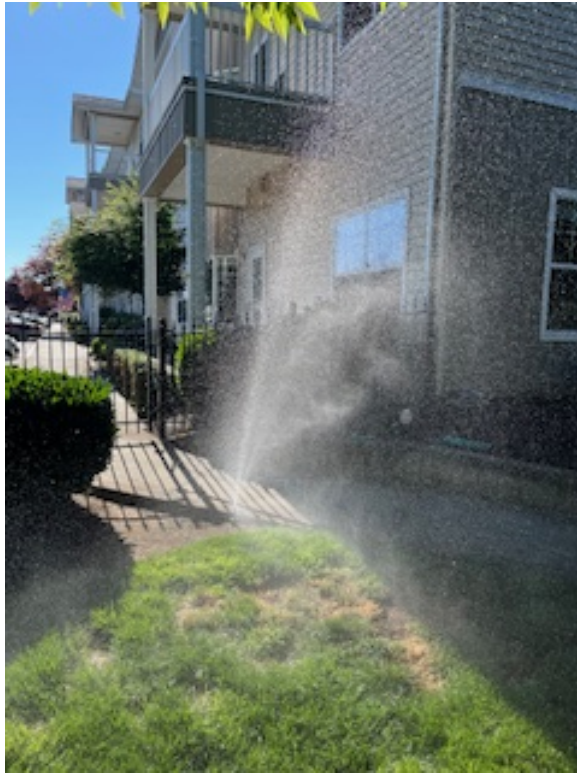
Broken Sprinkler Head
