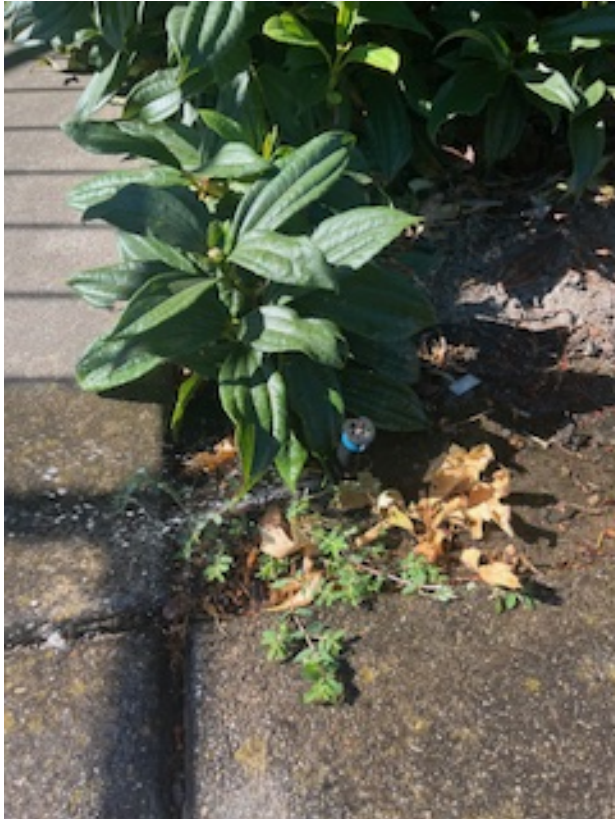
Broken Sprinkler head
