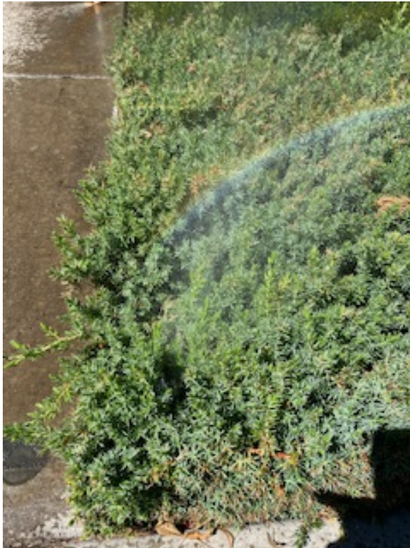
Evaporation from Blocked Sprinkler
