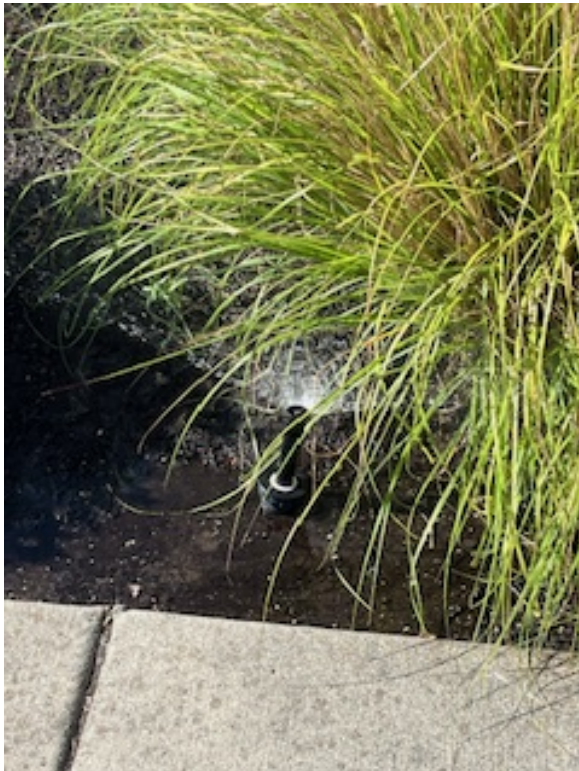
Blocked Sprinkler Head / Pooling Water
