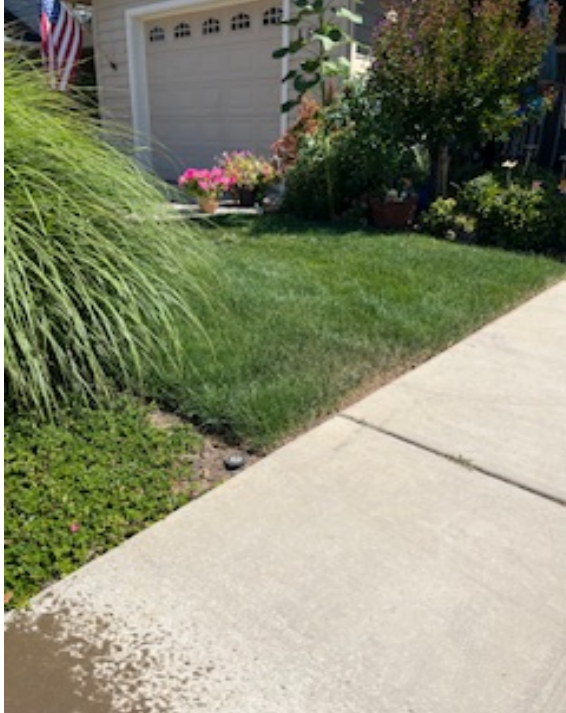
Sprinkler Head Not Working
