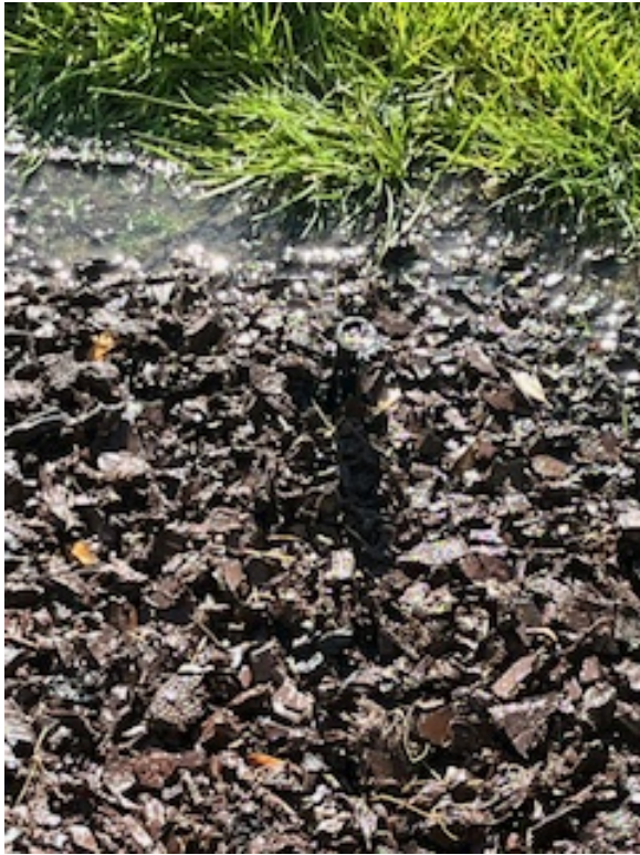
Broken Sprinkler Head
