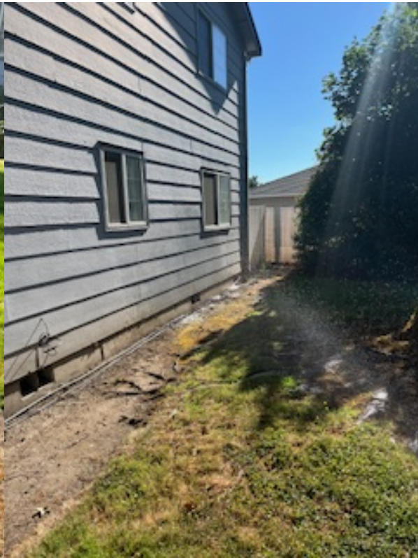
Spray hitting side of building into window
