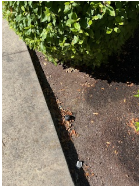
Sprinkler Head may be abandoned
