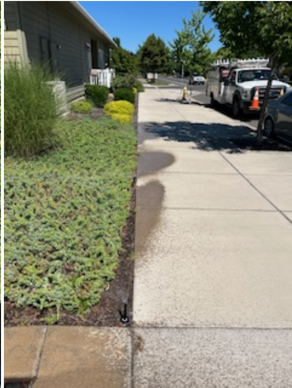
Alignment Needs to be adjusted
