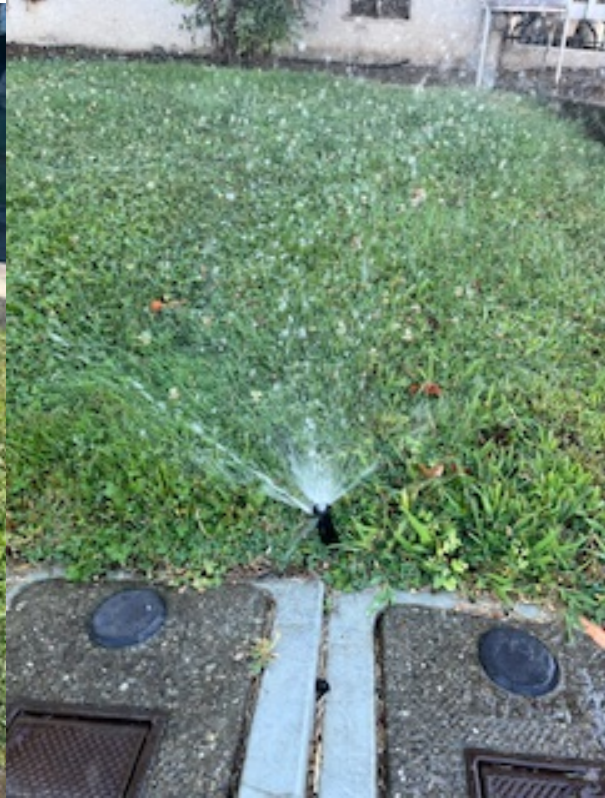
Broken Sprinkler Head
