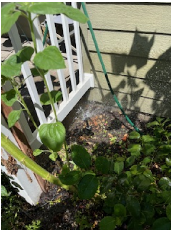
Broken Sprinkler Head
