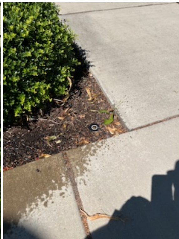
Sprinkler Head Not Working
