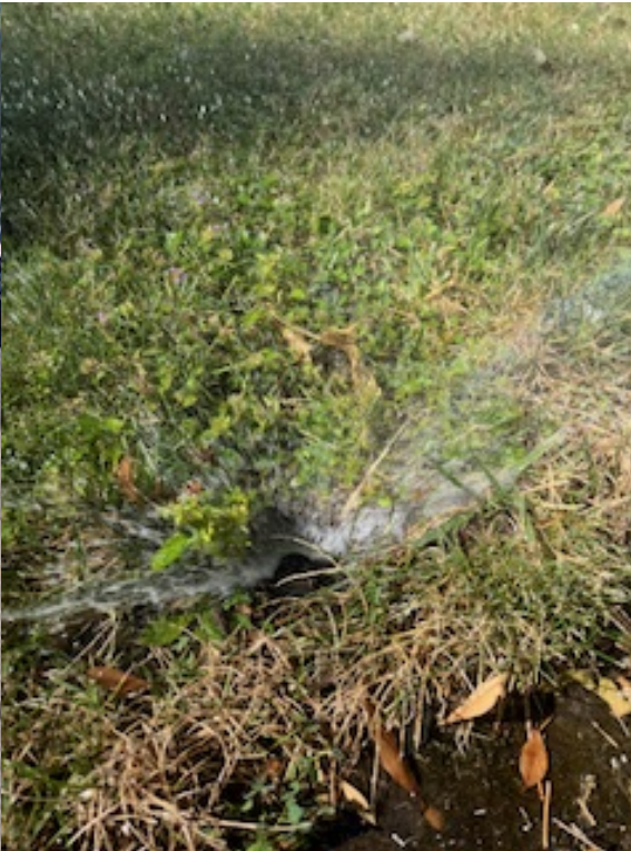
Broken Sprinkler Head
