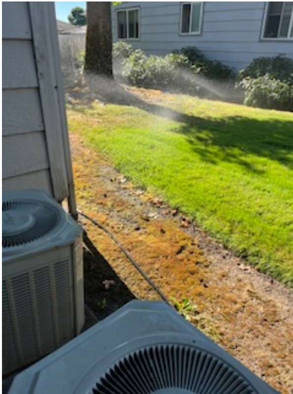
Spray hitting HVAC
