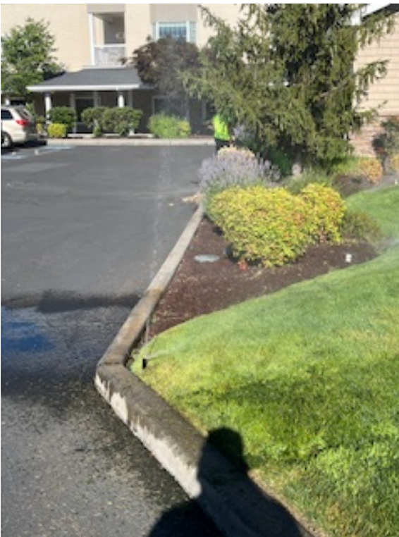
Broken Sprinkler Head
