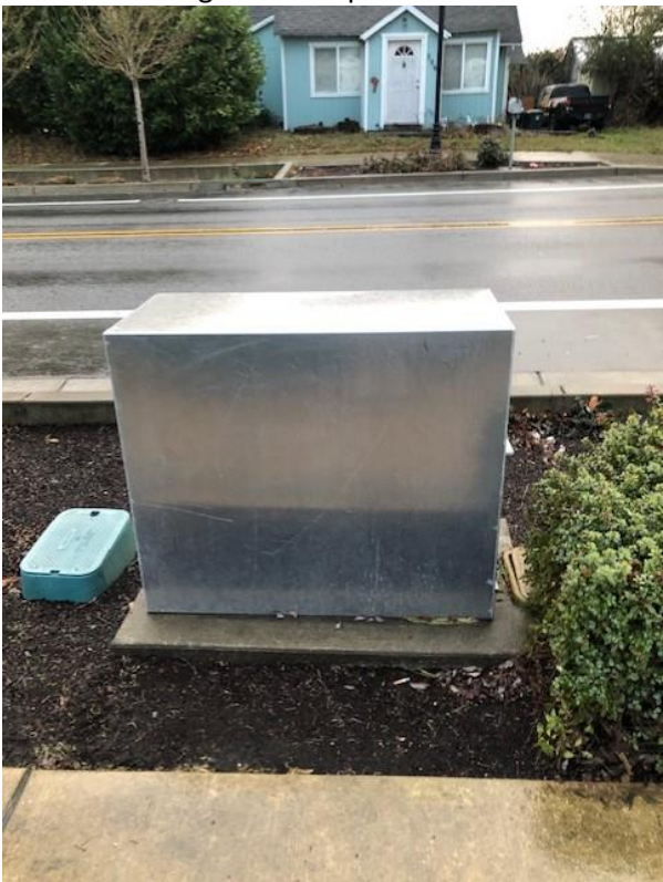
#11 S. Empire Blvd. North of WWTP #2 Width: 44" Height: 37" Depth: 20"
