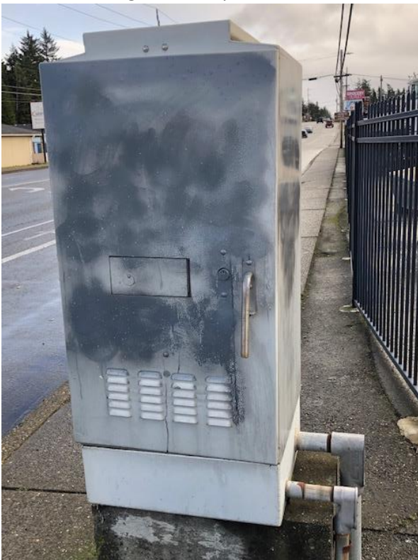
#3 At the Newmark-Ocean Blvd. "Y" Width: 24" Height: 54" Depth: 23"
