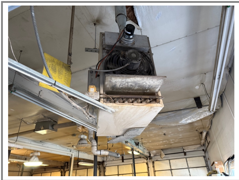
View of suspended heat system in north side shop building
