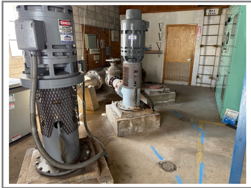
Interior views of 14' X 25' pump house in north shop building (not a part of appraised property SF)
