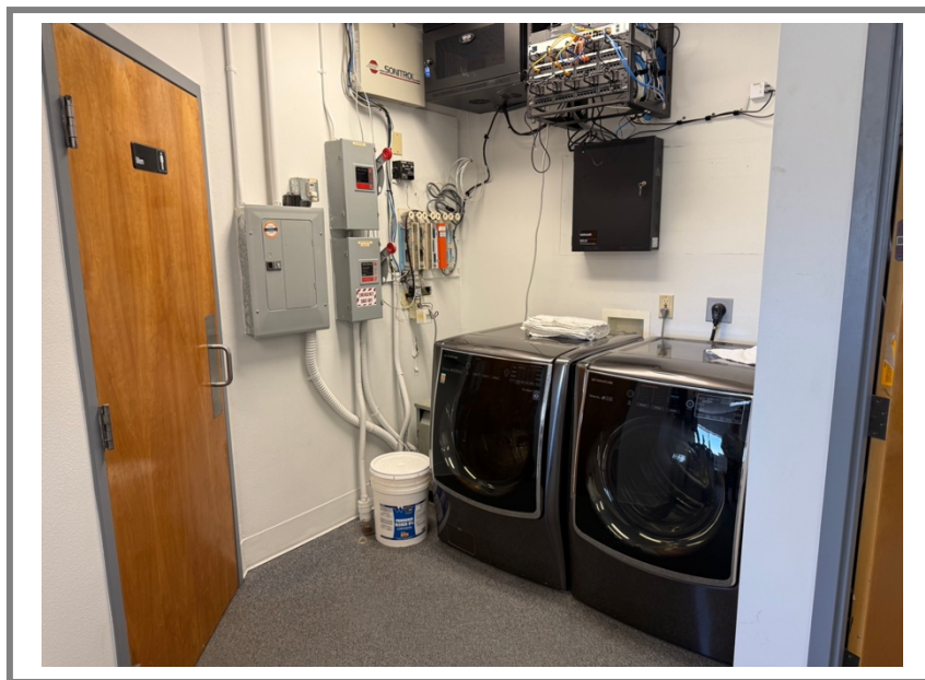
View of first floor laundry facilities in office building
